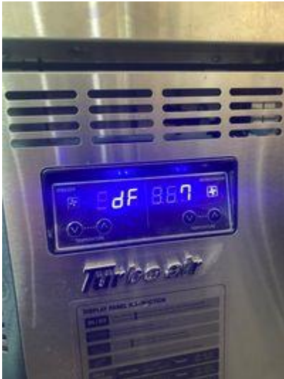
Ran unit in defrost mode all ok
